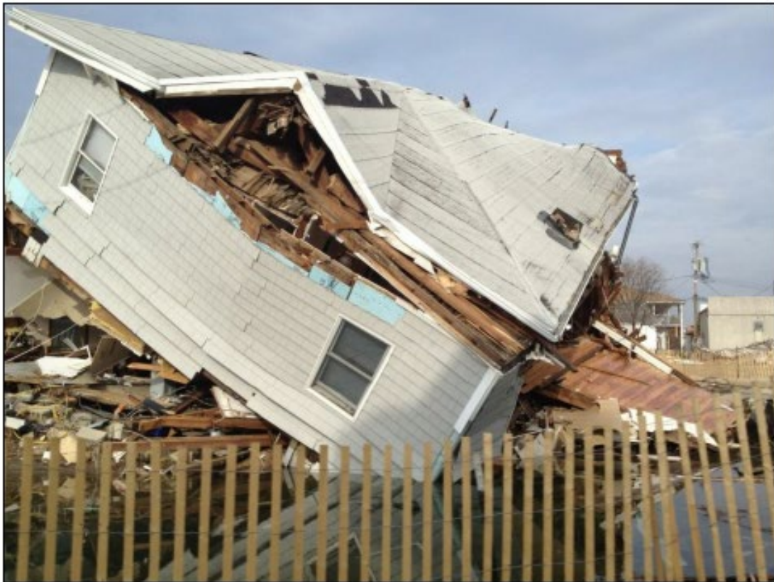
Image #4: The above example photo illustrates a building that is canted or wracked.
